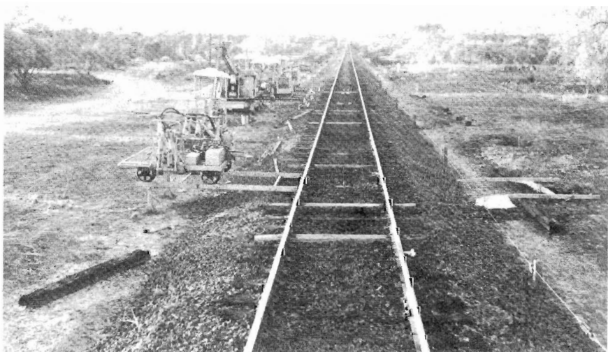
Track maintenance machines stand clear of the track at Hattah, between Ouyen and Mildura, during sleeper replacement operations after the bush fires.
